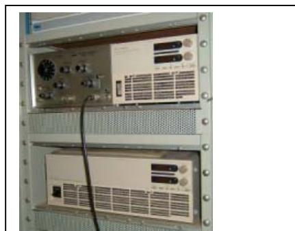
Fig. 7. Photo of power supply
